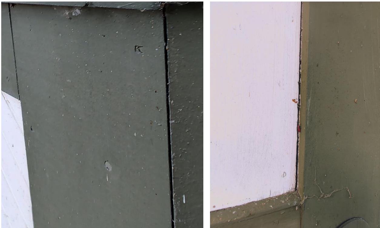
Views of existing gaps where existing trim boards meet and gaps between panels and trim boards.
