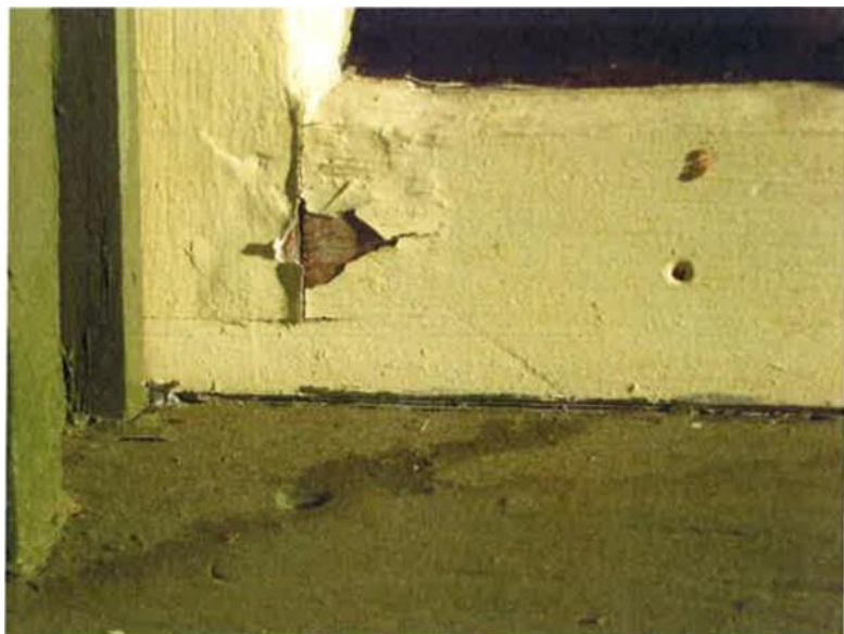
Peeling Paint at Window Sashes
