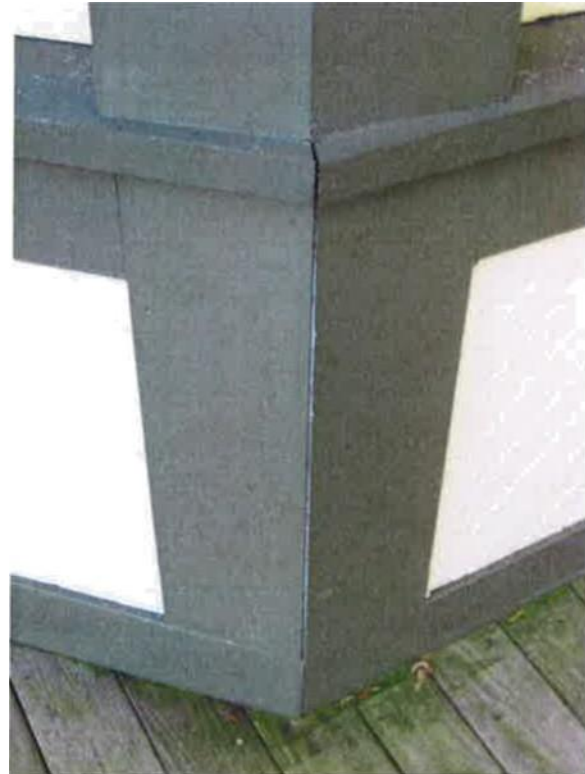
A Joint and Corner Board Trim That Has Opened
