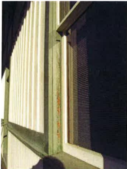
Peeling Paint at Window Jamb
