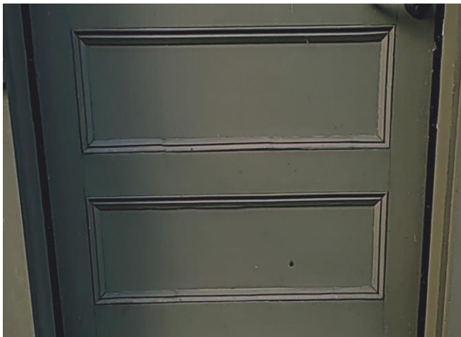
At some existing doors, molding at the panels have moved.
