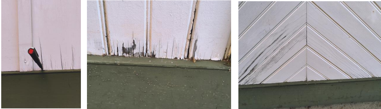
Views of existing cracks at the ends of existing trim boards and panels. New replacement to match existing
