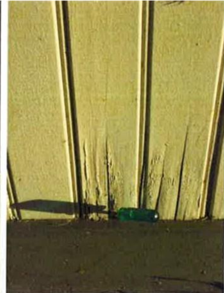
Painted Wood That Has Begun to Rot
